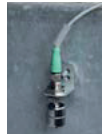
Filling level is monitored by probes
