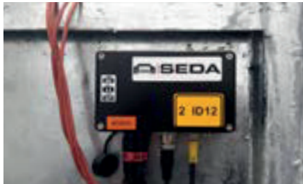
Monitoring sensors for each compartment
