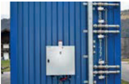
Control cabinet and water supply system
